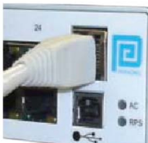
Figure 8: NIC Cable Connected*
